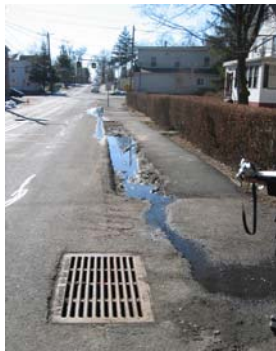
Surface Drainage Issues (Before)
