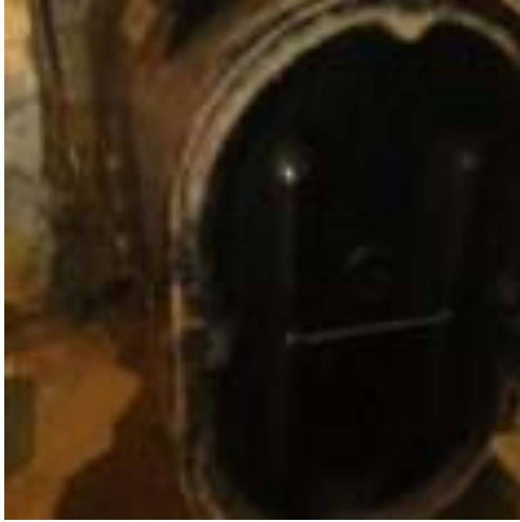
Photograph 13: View of heating oil AST in basement of Caruso residence (Parcel #1). View from south to north.
