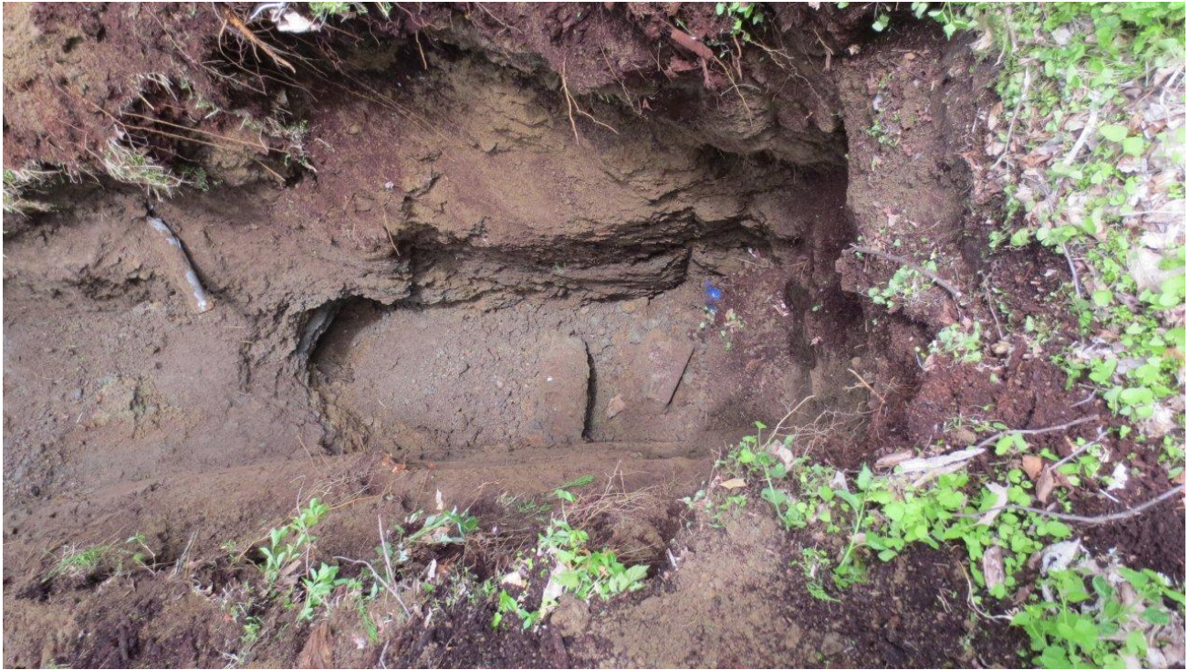
Photograph 11: View of the plastic conduit (left) and organic soil observed at TP-8.
