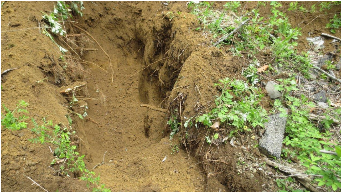
Photograph 4: View of surficial asphalt (right), dimensional lumber, and native soils observed at TP-3.
