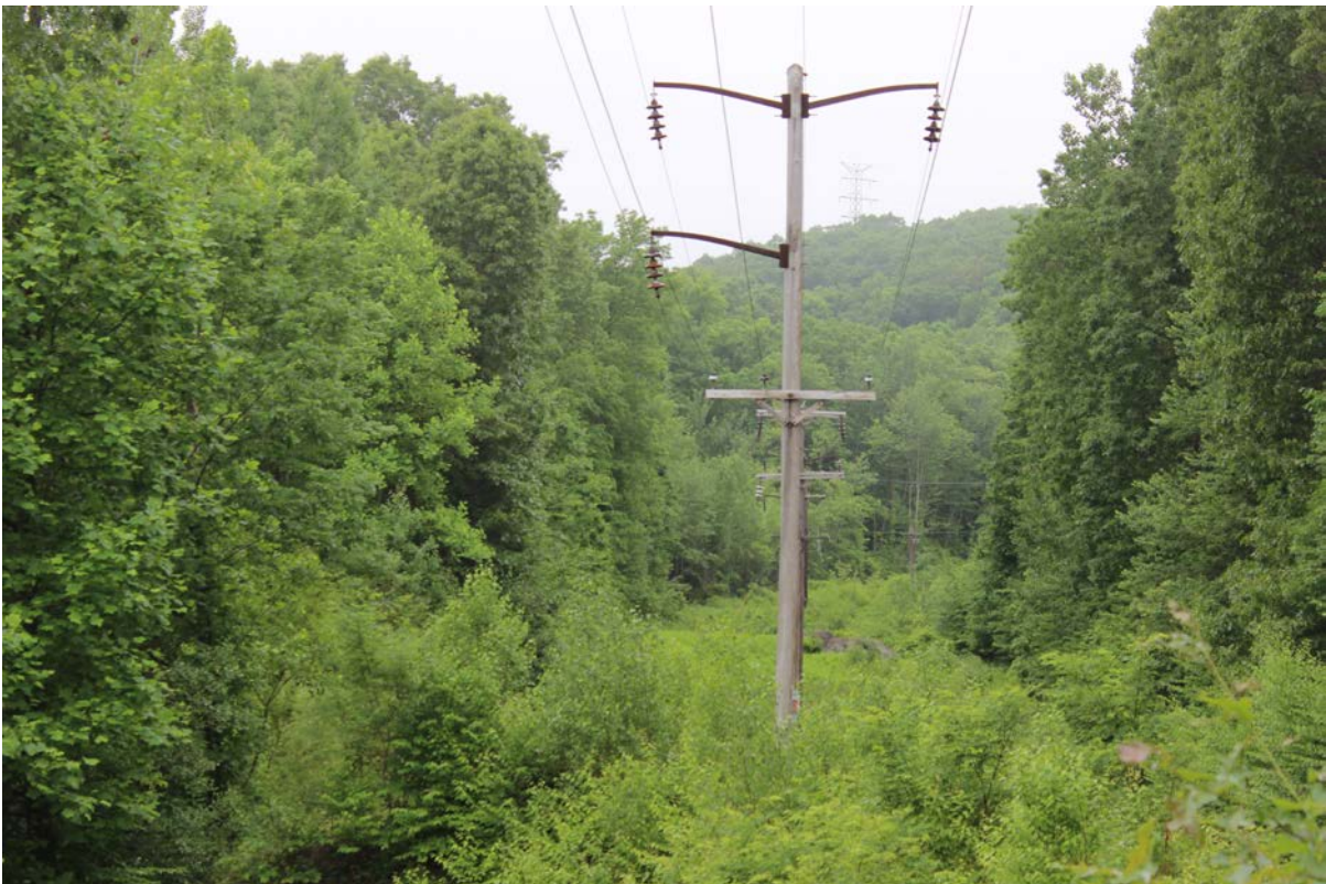
Photo 12 – O&R Transmission Line
