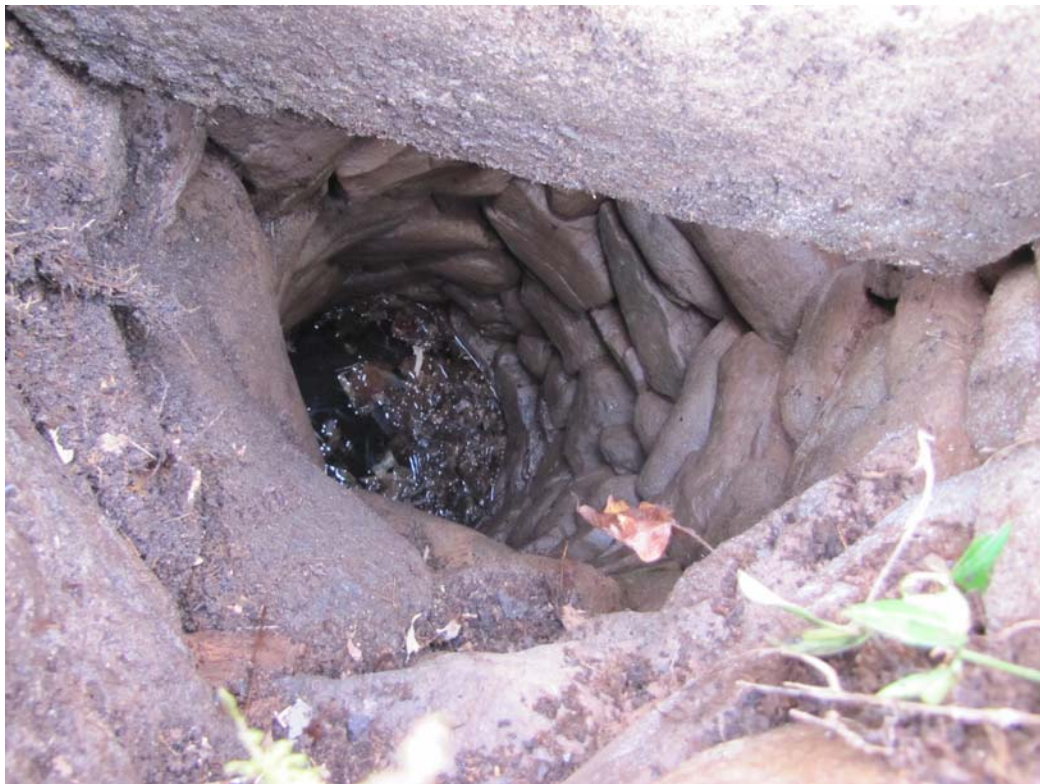
Photo 8: View into stone-lined well at southeastern corner of Clark Foundation. Water is at approx. 12'.
