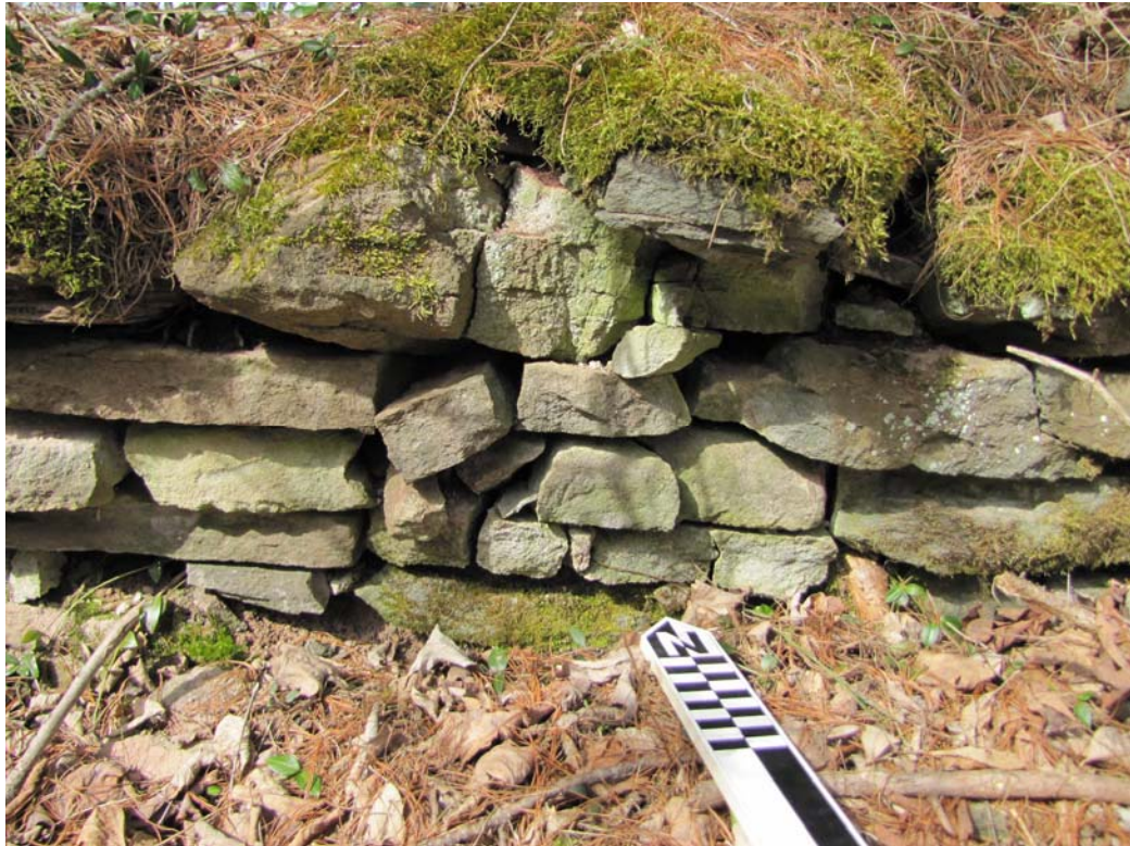
Photo 6: View north of interior face of upper course of Clark Foundation dry laid stone work.
