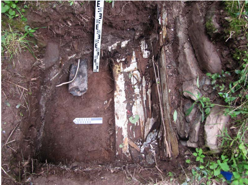
Photo 30: View of Unit 4 showing wooden panel door crushed against interior of foundation wall.
