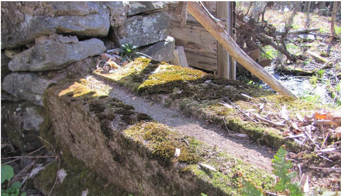
Photo 14: Photo of similar foundation wall and channel in D. Rumsey structure (MDS 7) north of test area.
