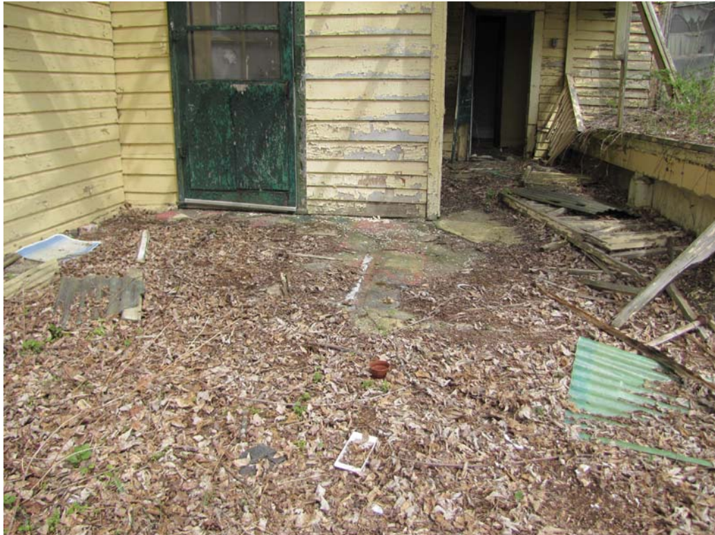
Photo 58: View north of concrete aprons outside rear doors of nearby Harvey Rumsey house (MDS 19).
