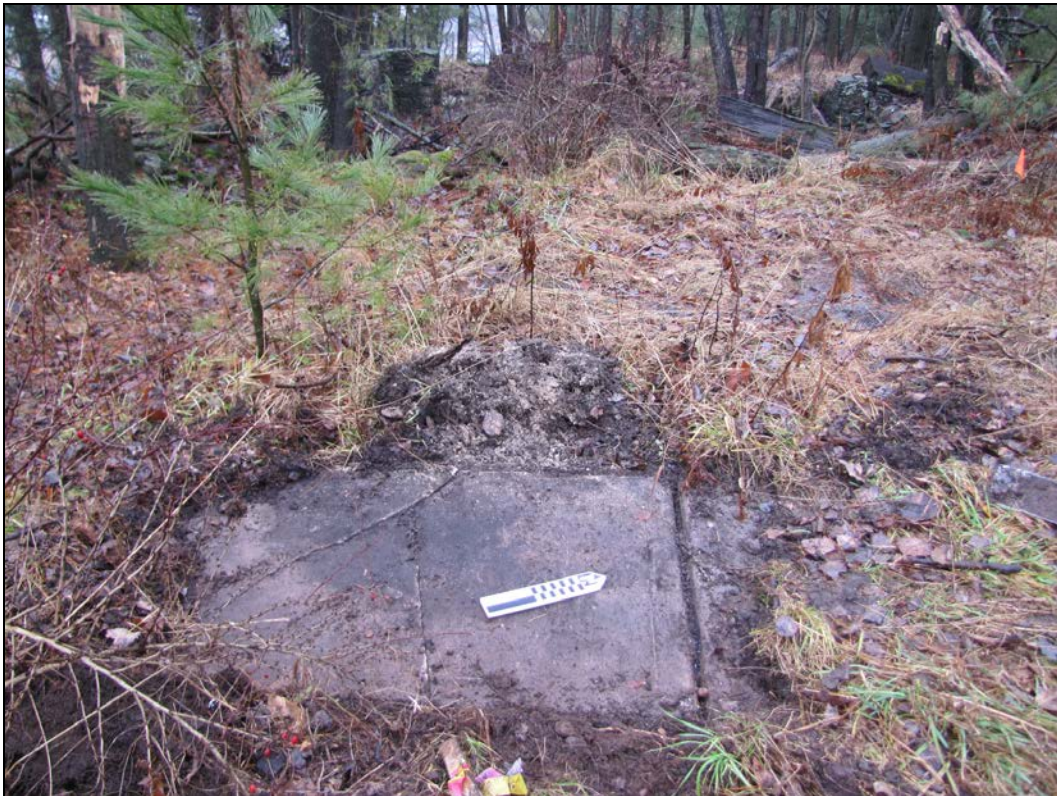
Photo 43: View west of Unit 13 location before removal of concrete sidewalk. Foundation is at rear.
