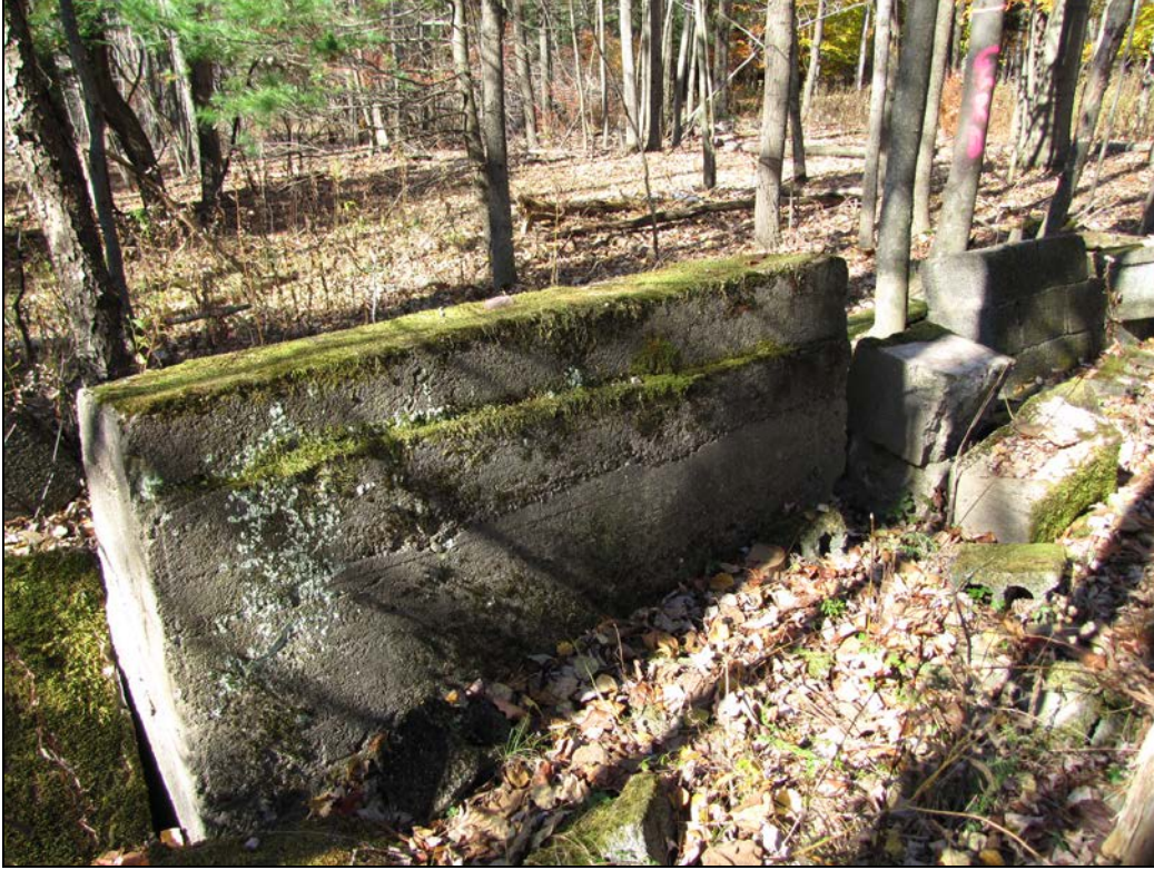
Photo 3: View west showing concrete foundation remains within Project Area west of Joyland Road.
