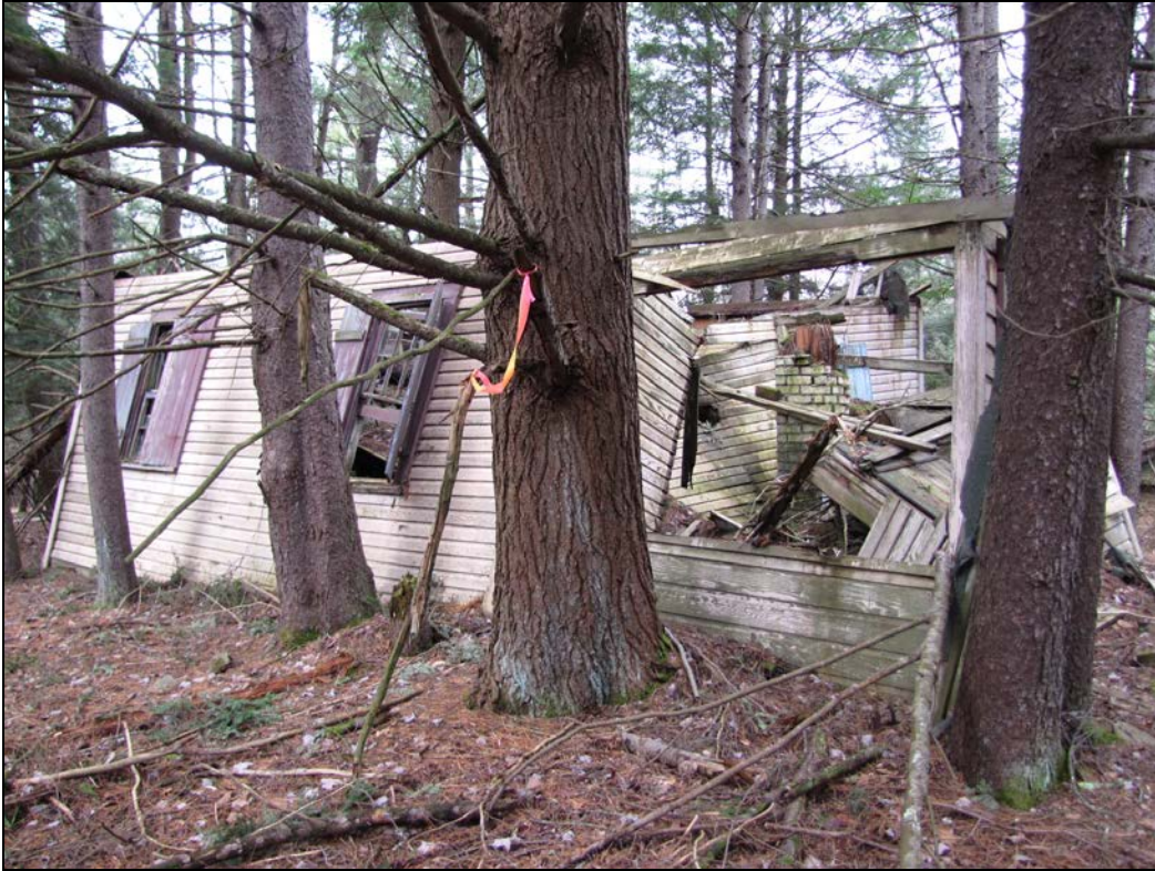
Photo 11: View southeast of second dilapidated cottage near Station 64+00 of roadway alignment.
