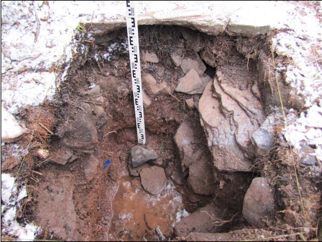
Photo 51: View east of Unit 22 with concrete sidewalk at top and foundation wall to right..
