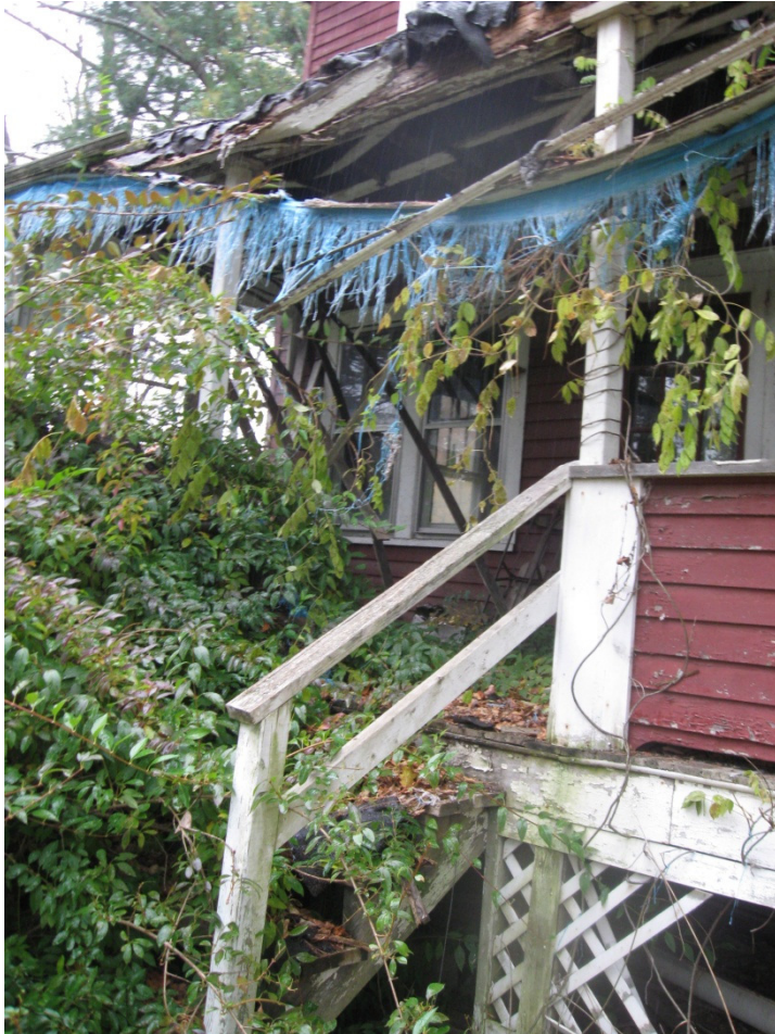
Detail of the collapsing porch roof.
