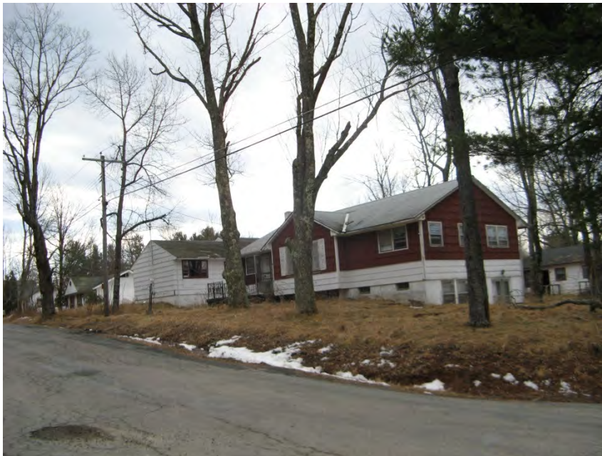
1. View southwest of bungalow colony, including three ranch style houses, at the intersection of Joyland and Thompsonville Roads.
