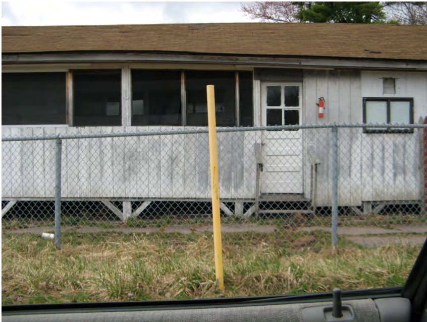
View of the east (Joyland Road) façade of bungalow building located on the north side of second northern driveway into the bungalow colony.
